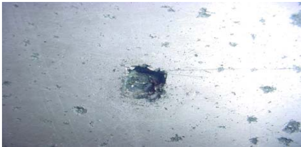
Figure 5 Typical problems with aluminium at sea is an electrolytic reaction causing omega pittings. These pitting vary from steel as they have extremely sharp edges and can develop inwards at an angle.
