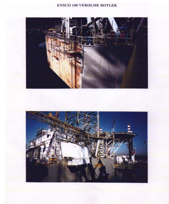
Figure 11 (above) The surface preparation was mostly hydro-jetting and the corrosion and poorly adhered
