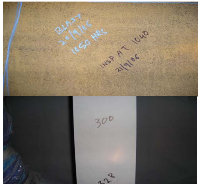
Figure 12 FPSO Enterprise required tank coatings which could be applied over UHP surface prep and rust bloom chose MCU Miozinc and MCU Mastic. The Miozinc displayed no mid cracking or blistering even when applied over 400% above the recommended dft.
