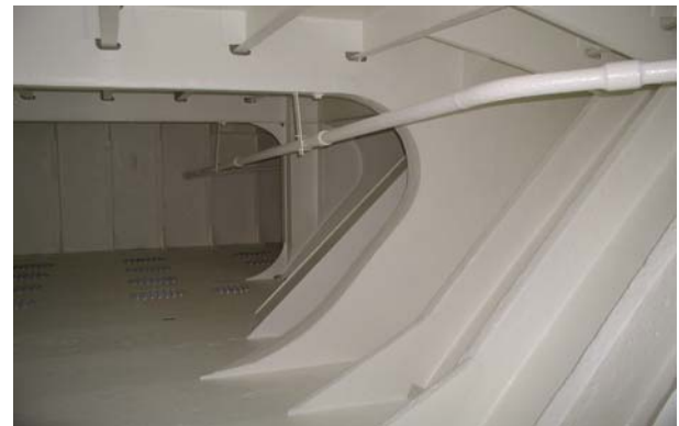
Figure 9 MV Hual Trubador, Ballast Tank, Hoegh Fleet Services AS. System: MCU-Miozinc – MCU-Mastic Completed by riding crew in 2000, water jetting surface preparation. After 3.5 years, the coating was 100%, with no breakdown and no signs of corrosion, even on edges and scuppers.
